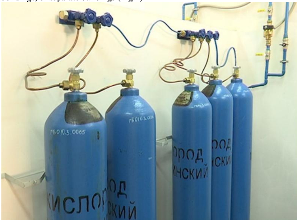
Fig. 1. Central oxygen point
